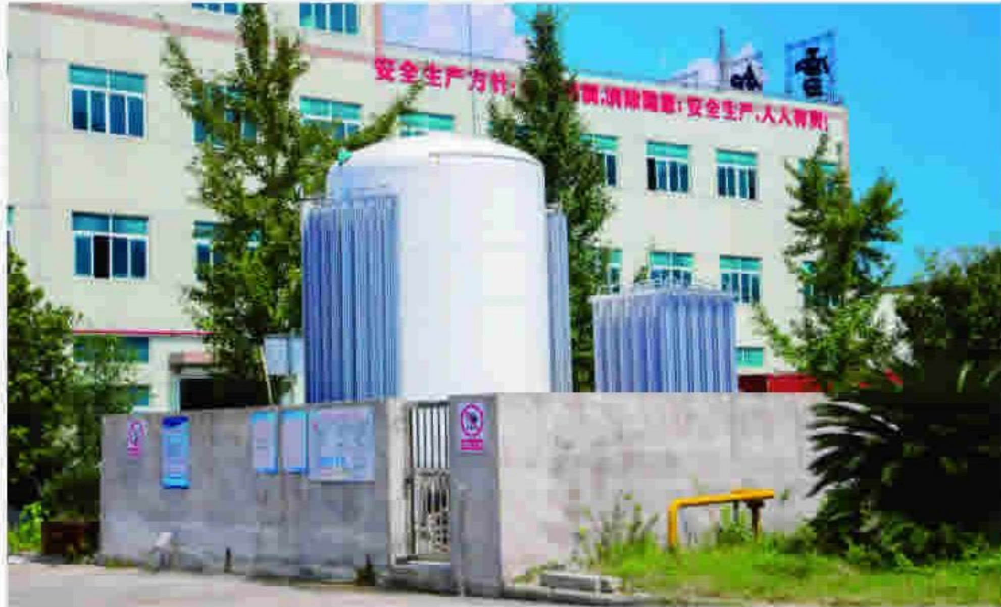
自建液化天然气站 SELF BUILT LIQUEFIED NATURAL GAS STATION
