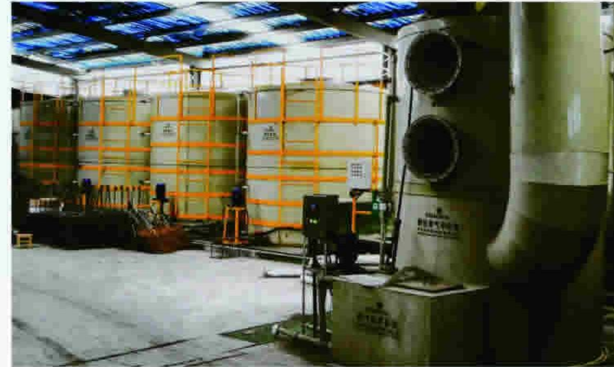
自建排放污水处理站 SELF-BUILT SEWAGE TREATMENT STATION
